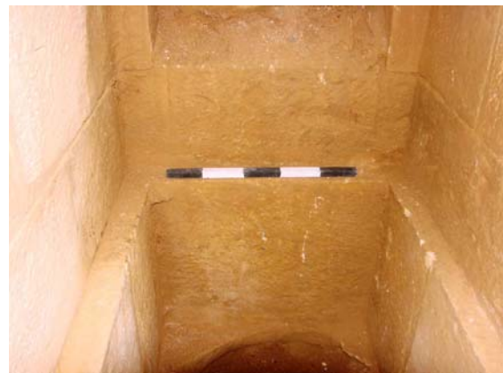
Figure 7a: photograph shows the edges of the vault upon which the side walls were constructed
