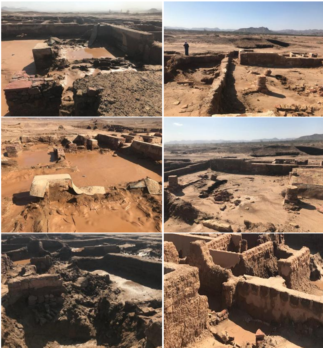
Figure 6. The Walls are Totally or Partially Destroyed by Natural Hazards and Erosion, Windstorms and Rainfall Mutually Influence Each Other, Resulting in Destruction of Mud Brick Features on Facades
