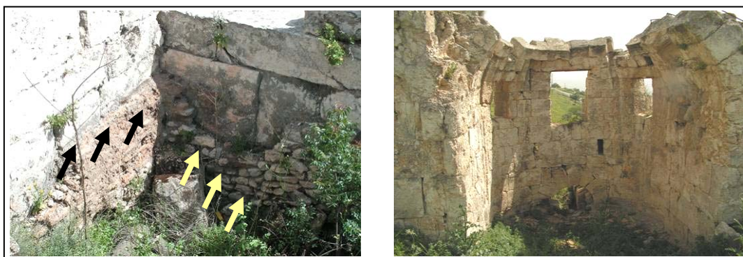
Fig. 3: Some physical deterioration forms affecting the brick structure
