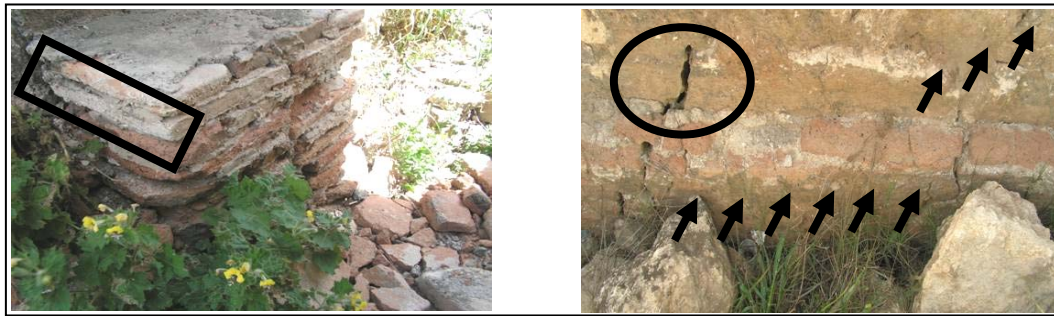
Fig. 5: Some biological deterioration forms affecting the brick structure
