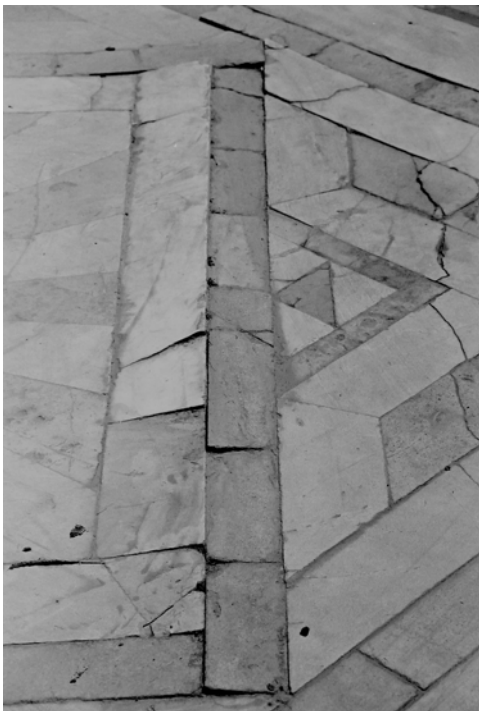
Fig. 4: General view of the severe deformations which affect the marble floor of the courtyard
