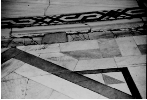
Fig. 3: Mortar of the setting-bed was altered to powder and dispersed on the surface of slabs causing their detachments
