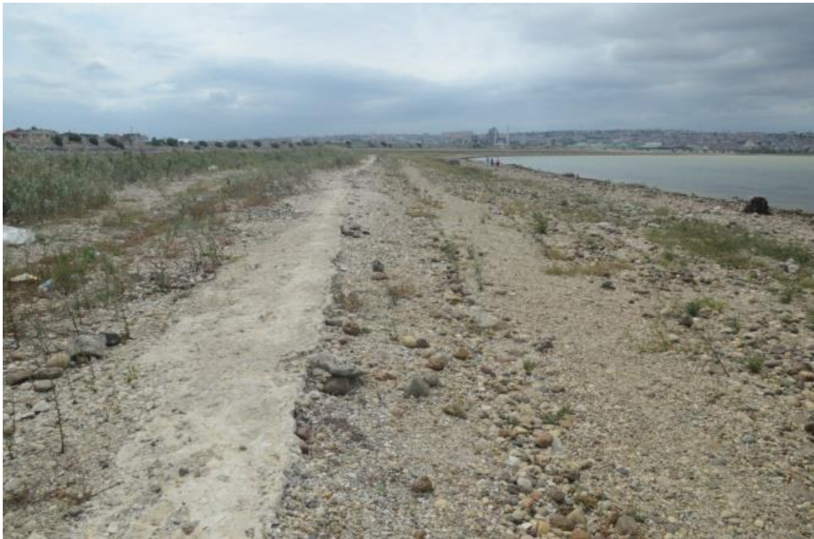
Figure 4b. A less obvious part of the embankment
