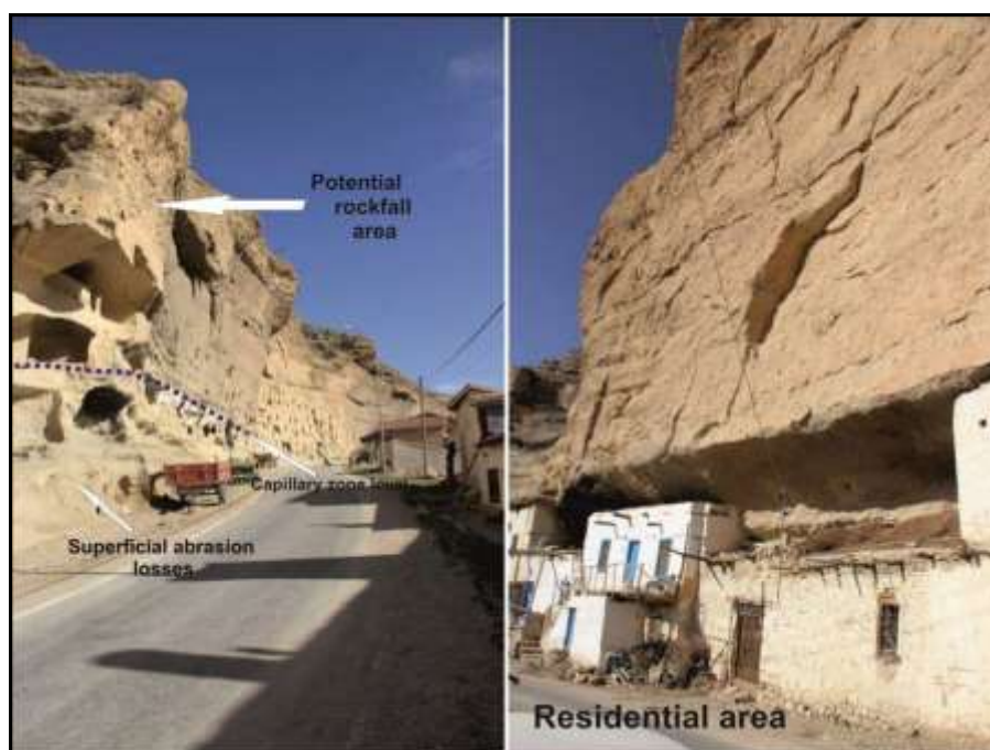
Figure 9. View of potential rockfall and residential area
