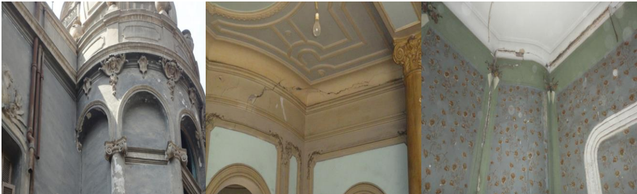
Figure.3a. present state of in plane and out of plane structural deficiency of Sakaini palace.
