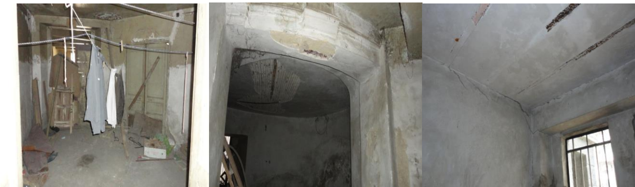
Figure.3b. present state of in plane and out of plane structural deficiency of Sakaini palace.
