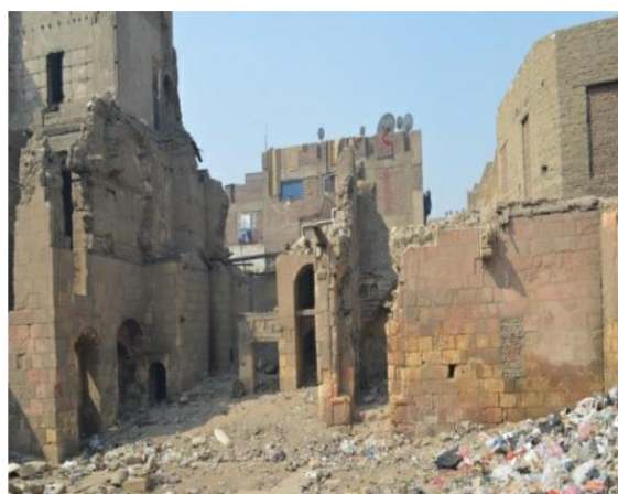
Figure 2. General view for the ground floor of Musafirkhana palace after fire.
