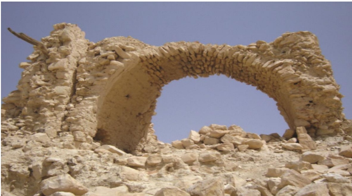
Figure 4. Arch structure at the site before collapsing.
