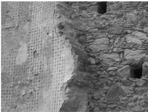
Figure 2: This picture clearly illustrates the use of "Caroselli" as structural element in the wall structure.
