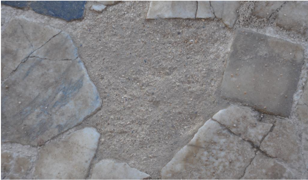
Figure 14. Old repairs made with ancient mortar.
