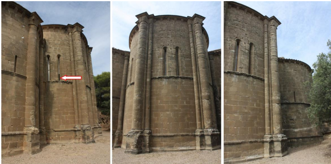
Figure 5.- Church of Santiago de Agüero. Apses with the situation of the windows.
