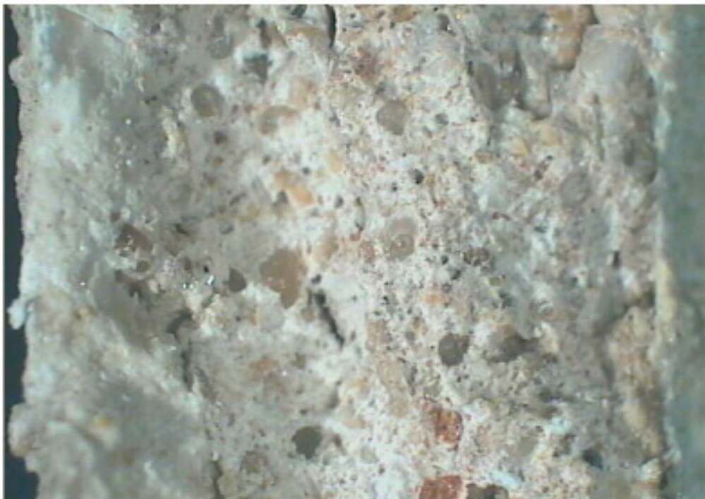
Figure 8. Well-compacted structural mortar with shrinkage cracks.
